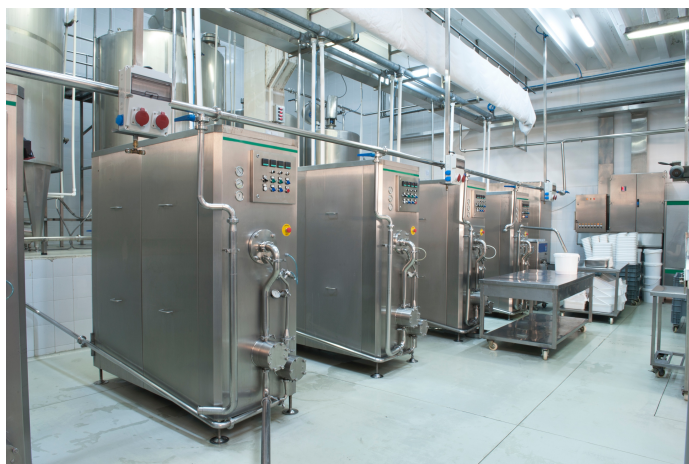
Pic. 9 Large production facility featuring 4 single cylinder continuous freezer.
